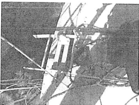
Roof exterior: showing bottom section of roof ladder equipped with the wheel assembly which is functional.
