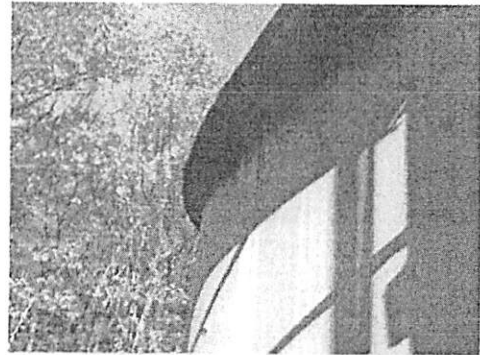
Shell exterior: showing rust staining weeping down from the unsealed roof to shell junction.
