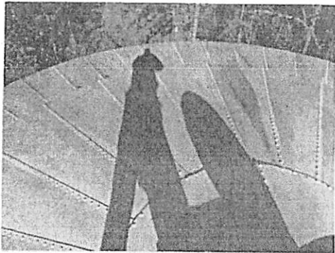
Roof exterior: showing existing coating to be in fair to good condition with only minor degradation and rusting taking place.
