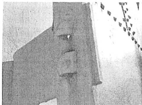
Shell exterior: showing additional degradation and rusting of the ladder side rail connections.
